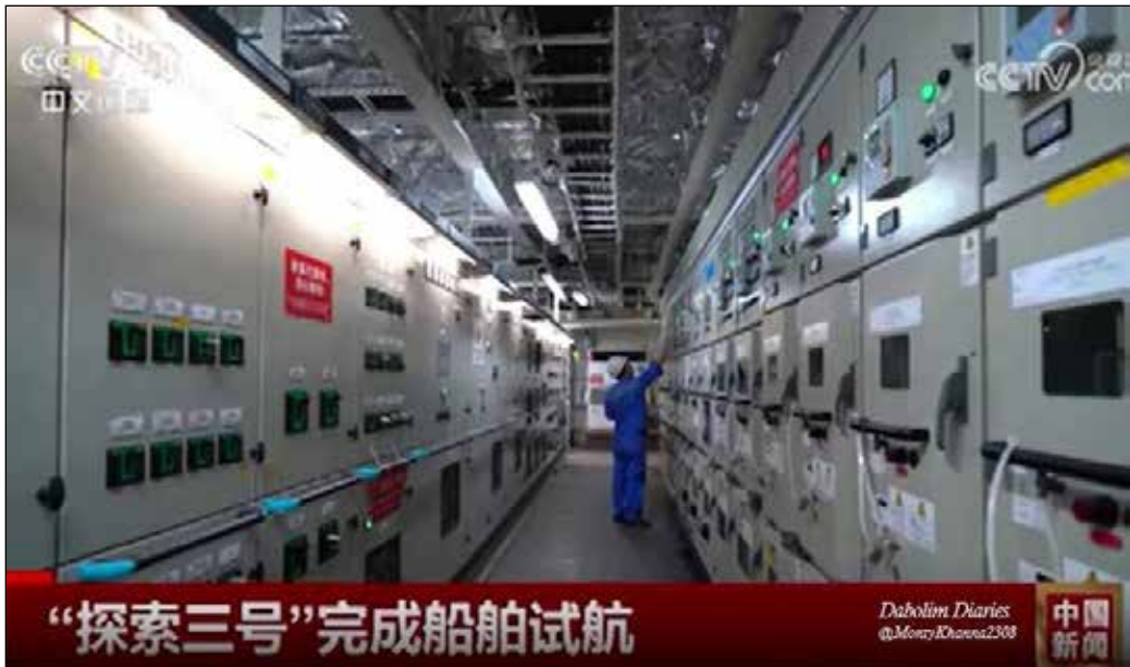
Figure 5: Electrical Power control room of Tan Suo San Hao (Exploration No 3)
