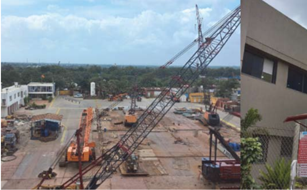
Figure 9. Geo-membrane layer on the yard and Liquid Oxygen supply tank in a yard Source: Pictures taken during the visit of Team NMF to ship recycling yards
